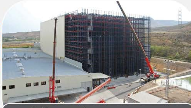
Self support (Rack-support building)
